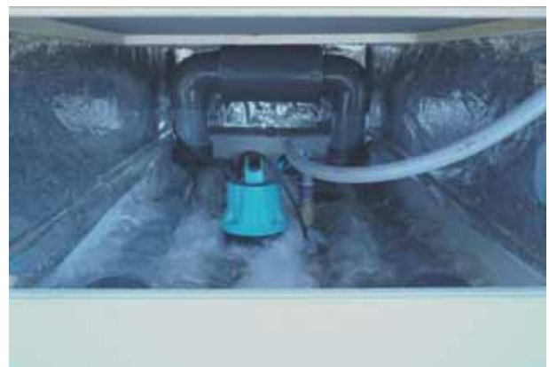
Fig. 3. The biofilter is equipped with an aeration chamber
